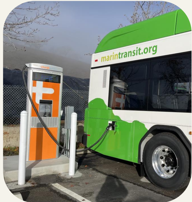
Bus Charging - Gillig Electric
